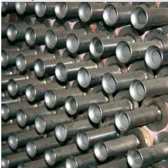
Ferrule at gas inlet tubesheet
