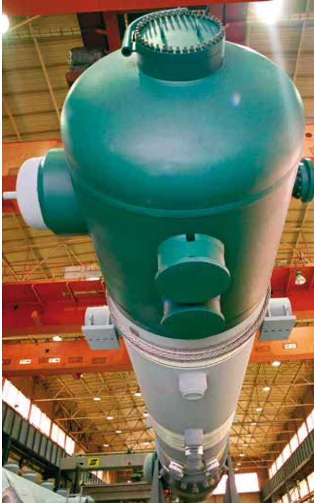
Process gas waste heat boiler
