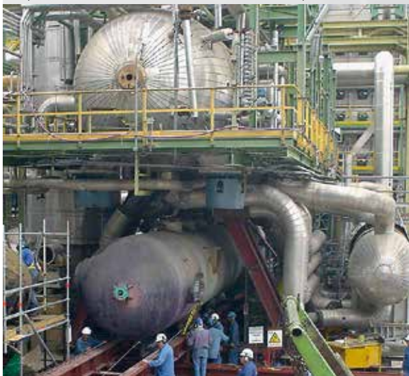
Replacement of a waste heat boilers under BORSIG supervision with mobilization of local personnel.
